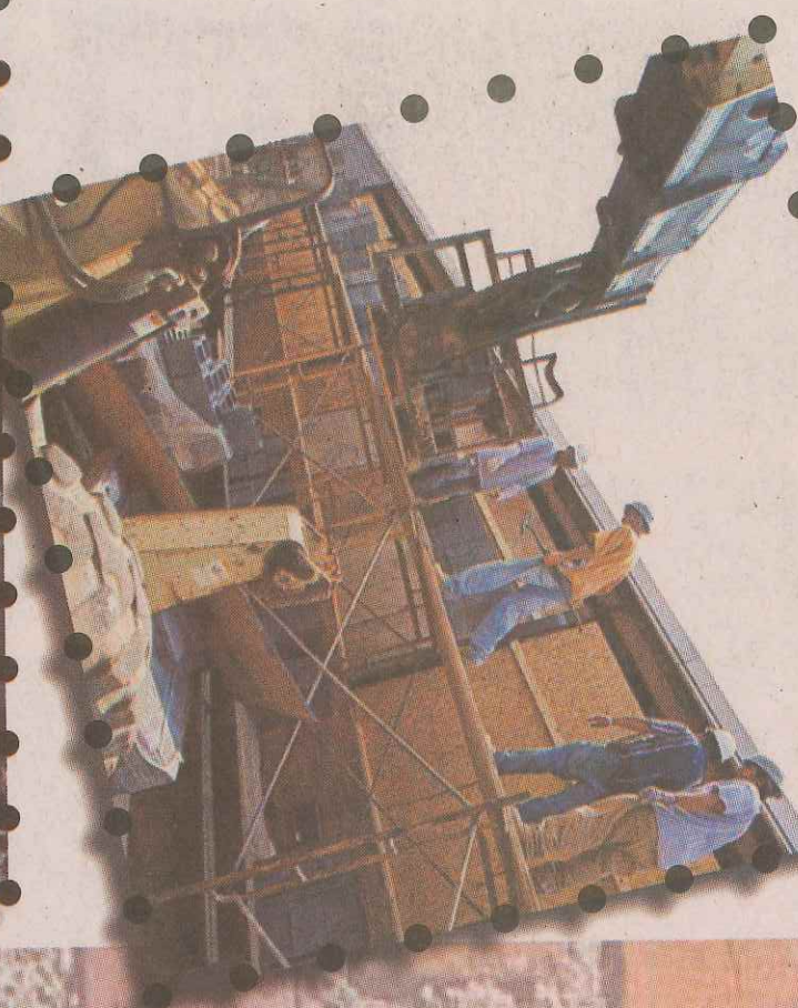
Thomas A. Edison High School in Alexandria, VA is being renovated right now.
